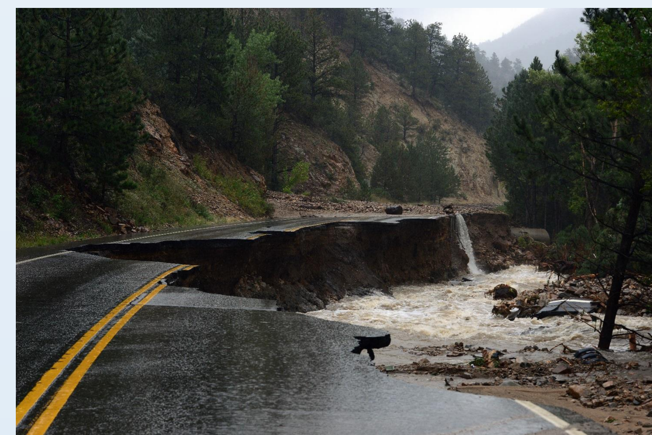
Flooding in Jamestown, CO.
